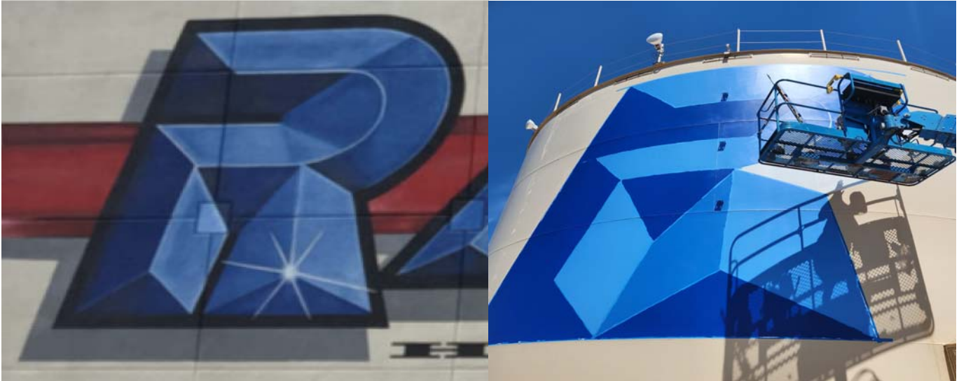
The “R” design on Robinson Tank matches the “R” in “Ramona” on the Ramona High School gym. Photo courtesy of RMWD.
